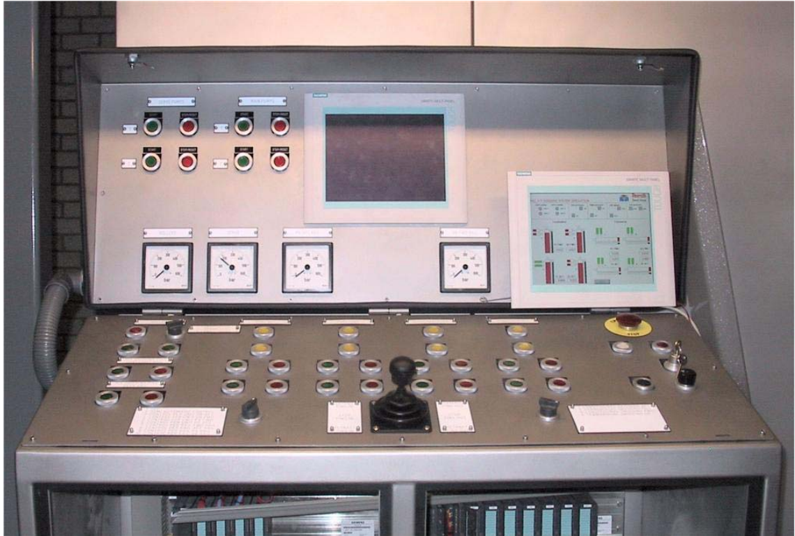
Figure 11: Skidding control desk
