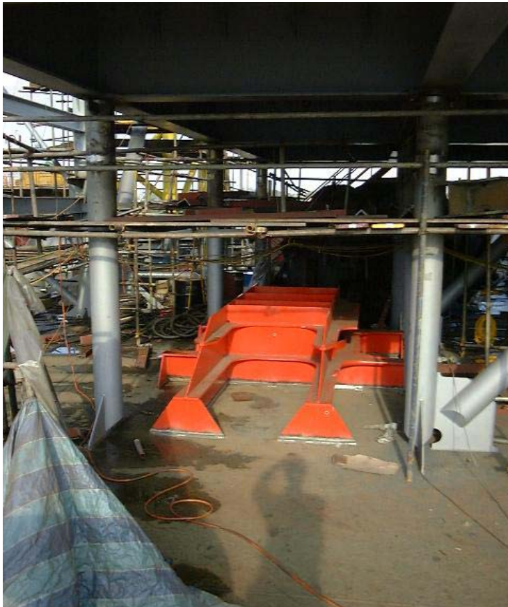
Figure 10 - Congested Deck Area for Spread Mooring FPSO
