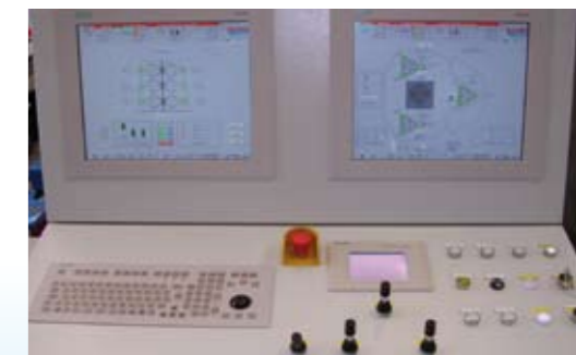
Central Control Console
